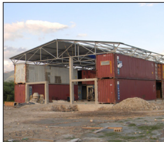
GAIN USA has built a warehouse from eight sea crates for storage of supplies and donations.
