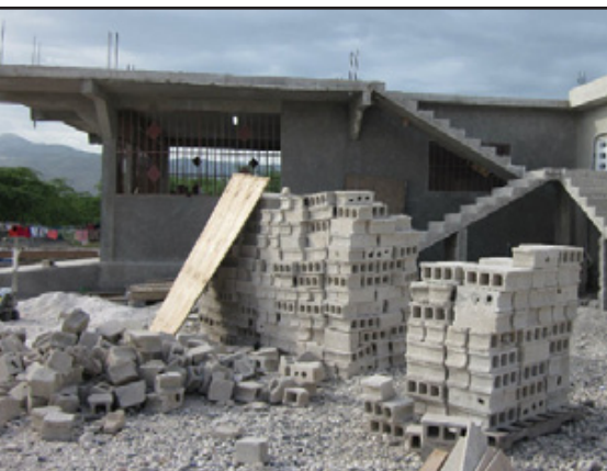
A second floor is being added to the preschool/clinic as result of your generous donations.
