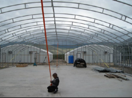
MercyShips is currently building a new community center on the Nehemiah campus. The two new volunteer dormitories are located next to it.
