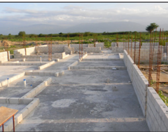
A new hospital is being built on campus thanks to the generosity of GAIiN, Mercy Response, Extreme Missionary Adventures and NVM volunteer teams.
