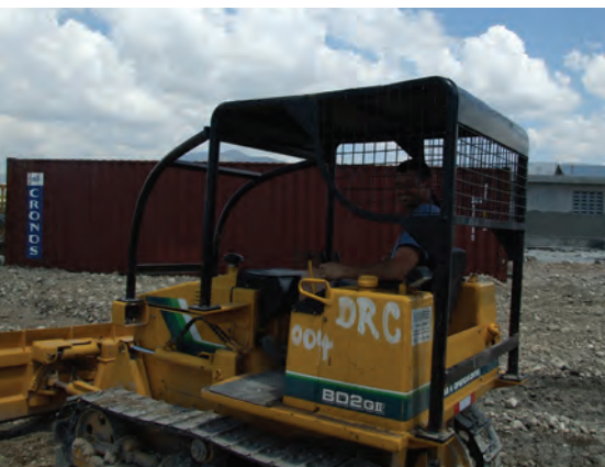
This small bulldozer arrived safely from Miami in early April and has made land preparation easier.
